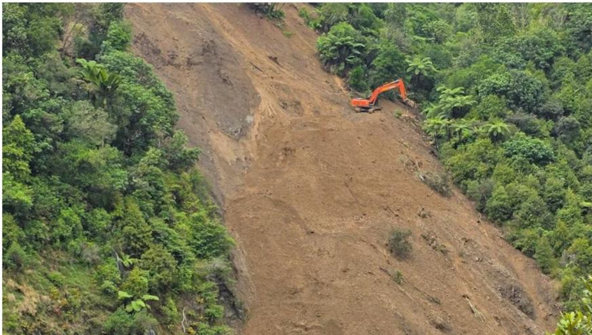
The Goldsmith slip on SH2. Photo / NZTA
